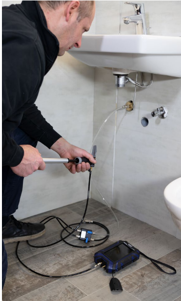
Fig. 53: Inflating the water pipe with air, the leak tightness test fittings are connected via stepped high-pressure plugs to the water pipe
