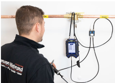
Fig. 21: Connection with the Wöhler leak tightness testing set for gas pipes for the stress test
