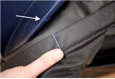
Fig. 9: Arrow indicates marking on the fan
