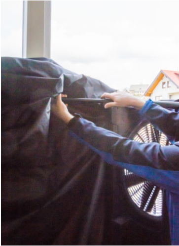
Fig. 16: Clamping the blower fan in a window with the telescopic rod
