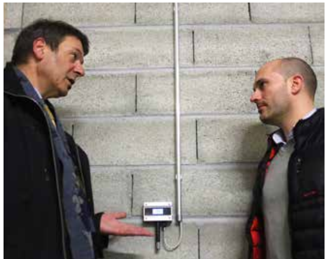
Marc Golay from Ports France Genève shows Marcel Rohrbach from Rotronic where one of the Rotronic transmitters is mounted.
